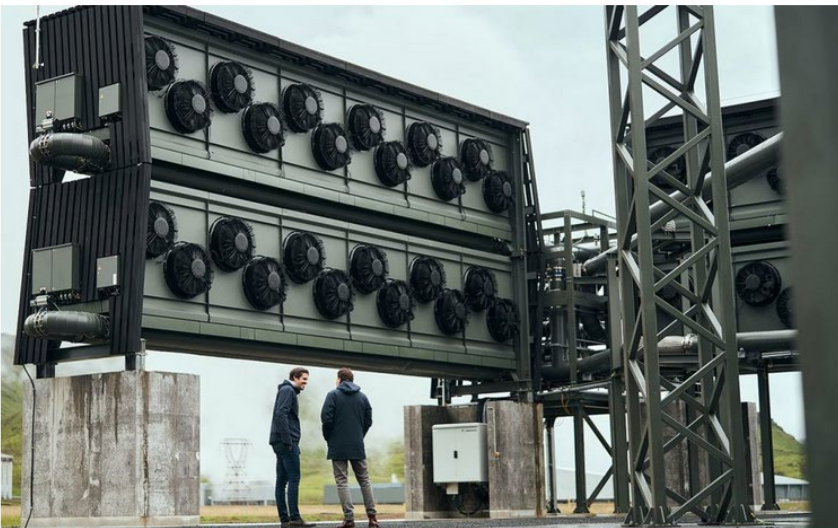
Orca CO 2 direct air capture plant in Iceland (source: Climeworks)
